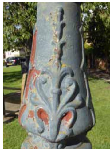
Figure 84: Street lamp requiring repainting, Little Green
